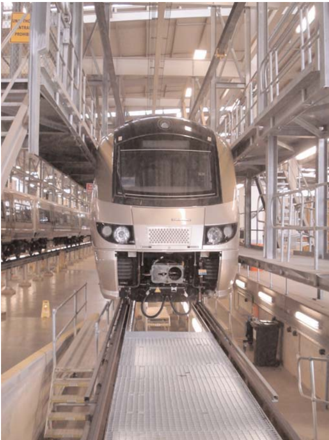
Figure 6 Gautrain car in the depot.
